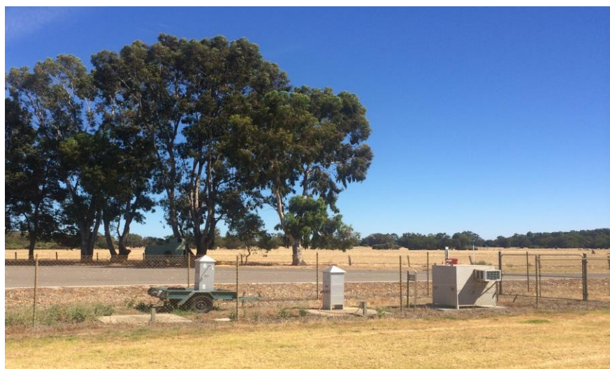
Figure 7: Dust Sampling Equipment at Pinjarra Racecourse (including spare trailer-mounted HVAS unit)
