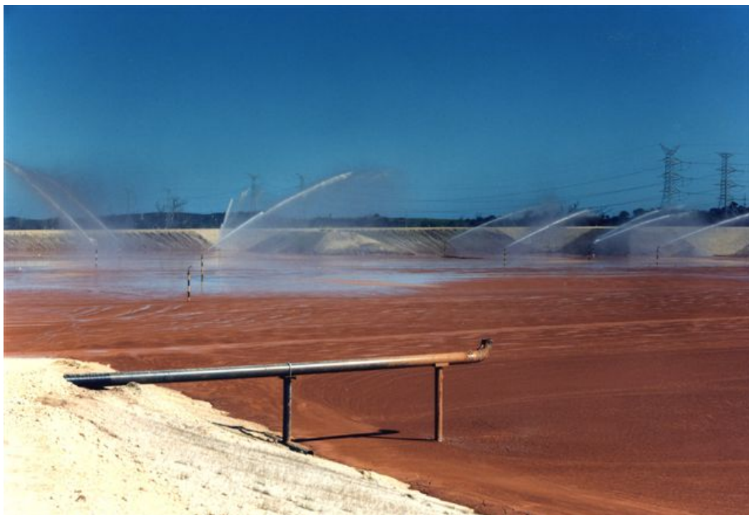
Figure 1.4 A Residue Drying Area (Kwinana) showing pipe from which residue is poured, with operation of water cannon in background
