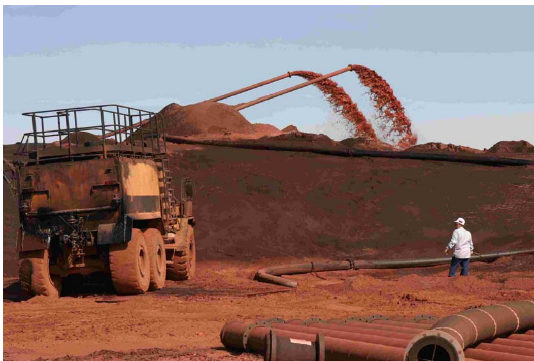
Figure 1.8 Sealing of sand stockpile area with bitumen emulsion. The Sand slurry is being pumped into the stockpile in the background
