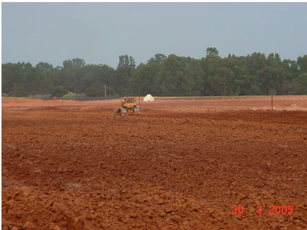
Figure 1.7 Operation of dozer on “dry” residue levelling the residue in preparation for the next “pour”
